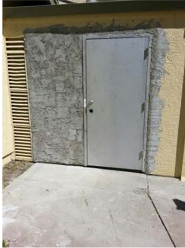
New Equipment Room Door at May Valley Community Center
