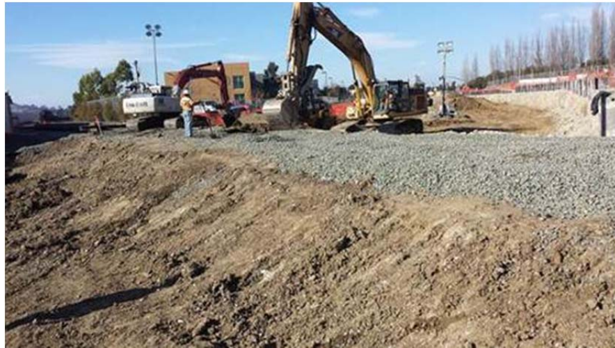
12:30 pm Saturday, December 14 th , tracks removed and beginning excavation to reveal precast abutments placed in November
