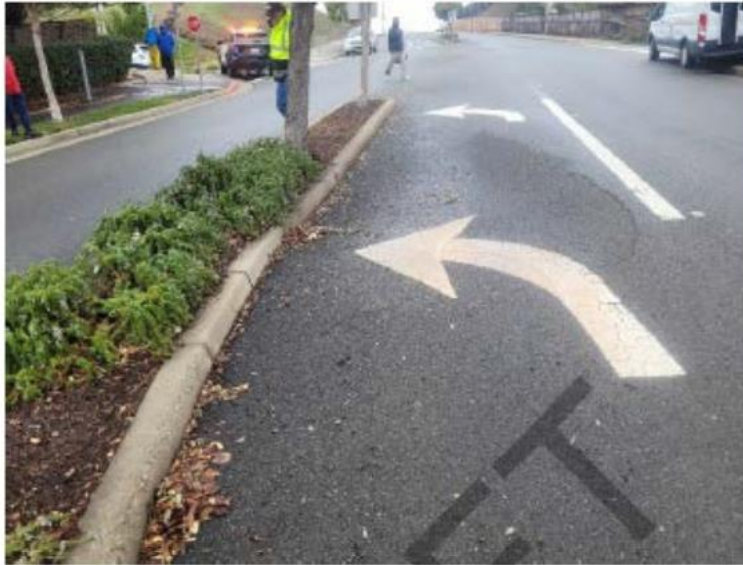
View of depression and cracking in asphalt on Seacliff Drive.
